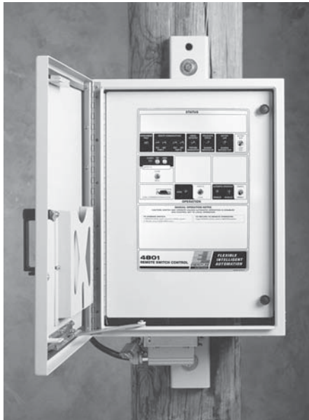
New EnergyLine 4801 Remote Switch Control
